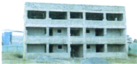
Construction of International and Training Centre Unit for Research Centre and Start-Up Village Centre Phase II
