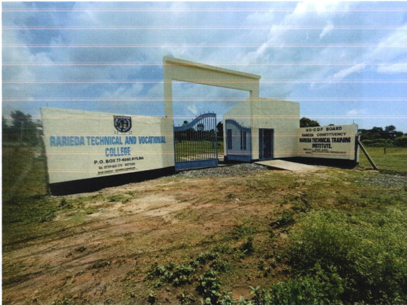
Figure 12: Fencing and Installation of A gate at Rarieda Technical and Vocational College
