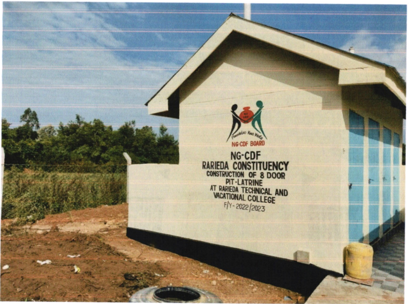
Figure 10: Construction of 8No. Door Pit Latrine At Rarieda Technical And Vocational College
